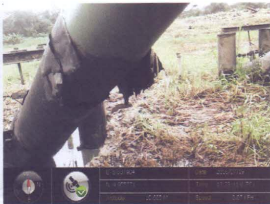
Picture of the dented pipeline.
